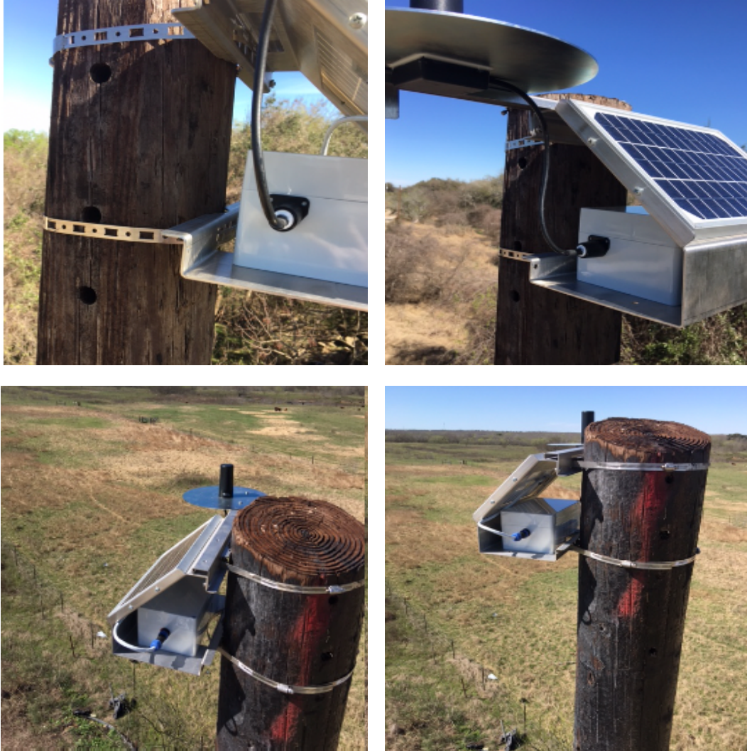
Figure 2: Completed Installation of Allegro AC Repeater
